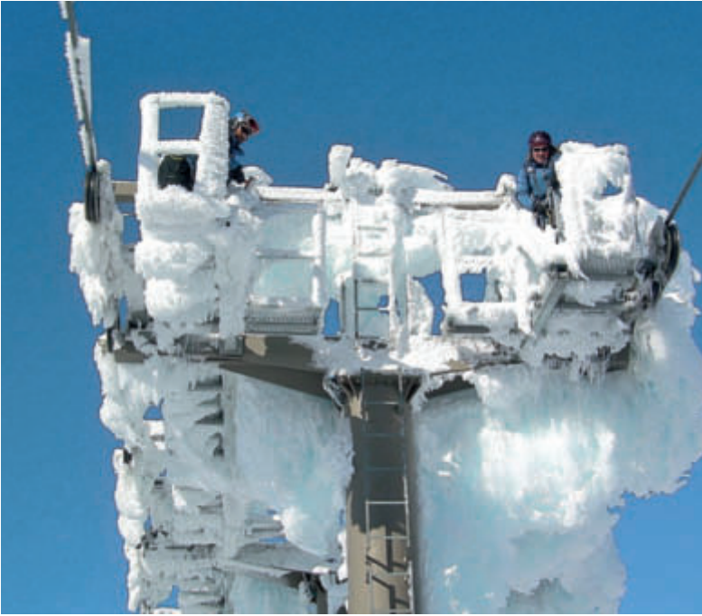
Tower head completely enclosed in ice
